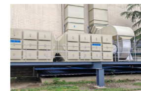
Waste Gas Treatment Equipment at Xindu Base Workshop
