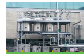
Dichloromethane Waste Gas Treatment Facility of Yueyang Branch
